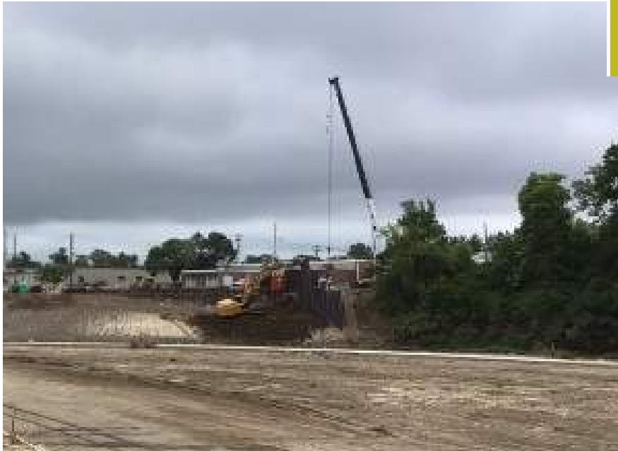
Phase I remaining sheet pile wall installation south of Deer Creek near Exchange Way.
