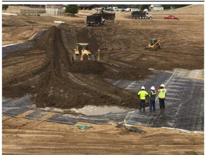
Phase I cover soil backfill and grading for the clay liner installation at the large Pond near Mary Ave.
