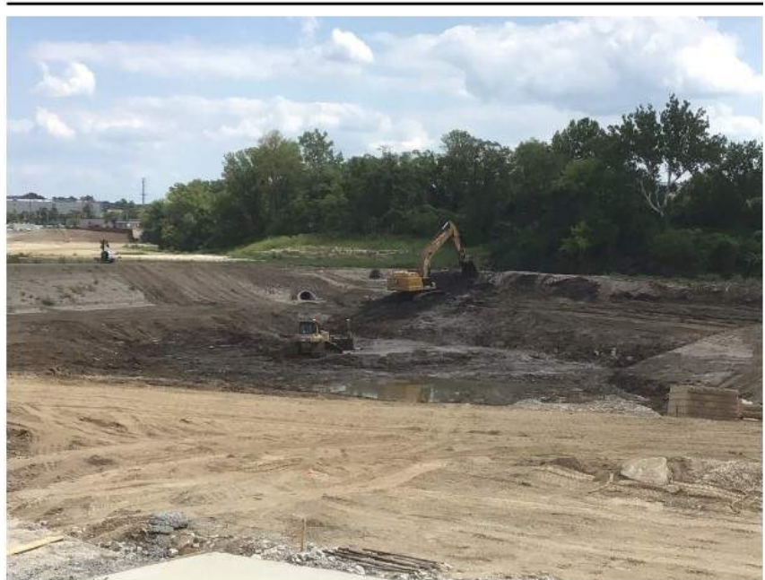
Phase 1 silt removal at the large Pond near Mary Ave following dewatering from the flood event early Aug.
