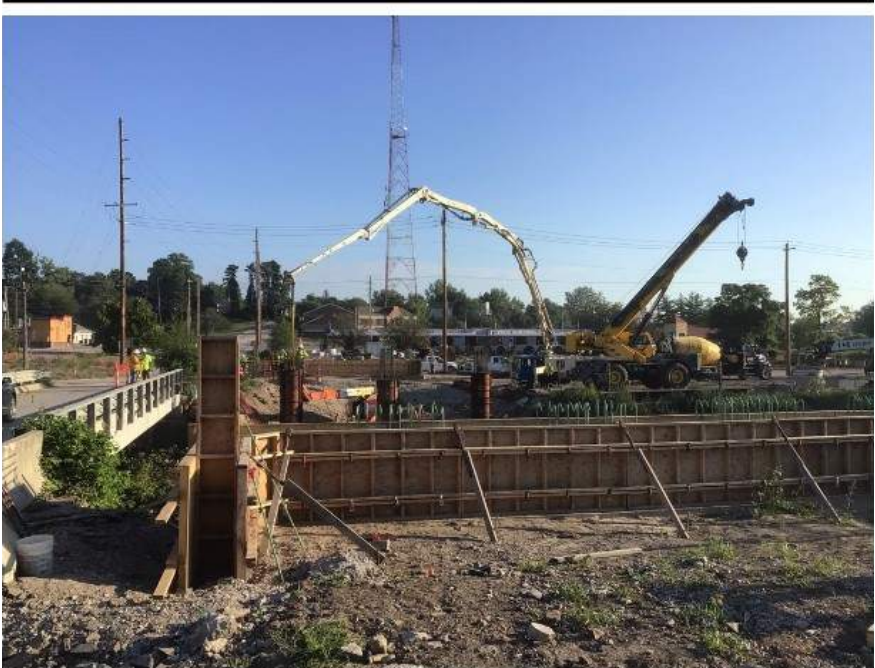
Phase II concrete pumping for the Breckenridge Ind. Ct Bridge intermediate and end bent construction.
