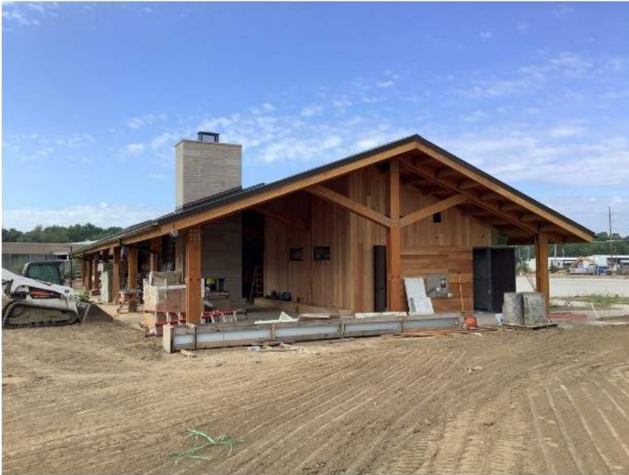
Comfort Station (Pavilion) structure south elevation completed wood siding near the fire place area.
