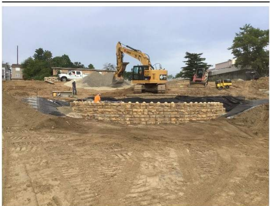
GRG Connector Part A amphitheater retaining wall construction at the large Pond near Mary Ave.
