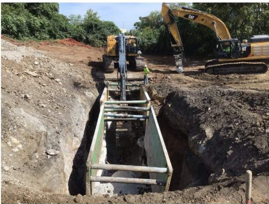
Phase II 72" sanitary sewer excavation and piping installation north of Manchester Rd.
