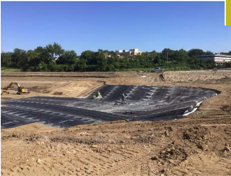
Phase I installation of the geosynthetic clay liner for the large Pond near Mary Ave.
