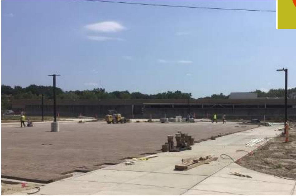
GRG Connector Part A installation of permeable pavers for the parking lot west of the Pavilion.
